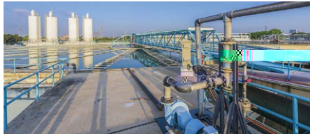
Water Plant Retrofit & Upgrade
